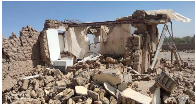
Figure: The damaged house in Wardak Ha was taken from the Un website
